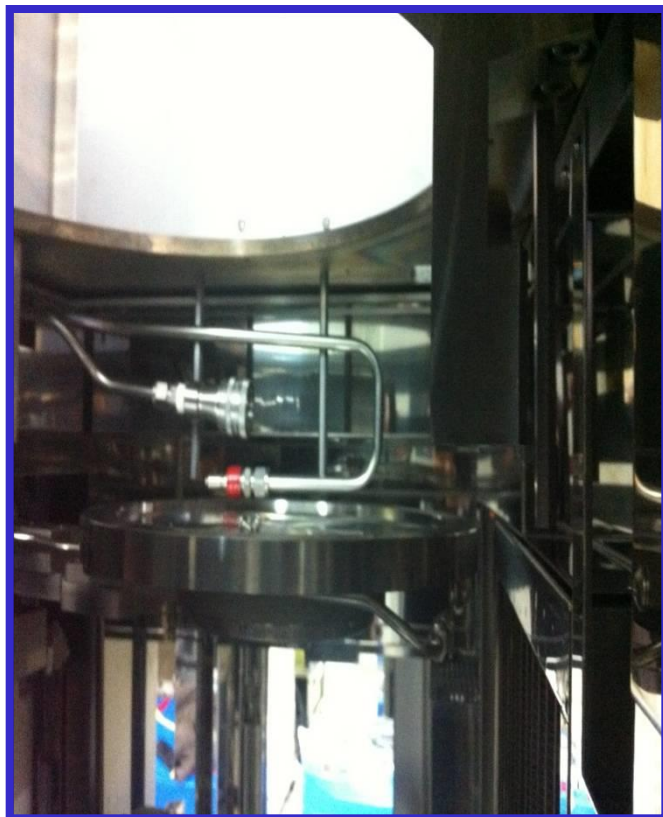
Flange PCW Line (Exchange)
