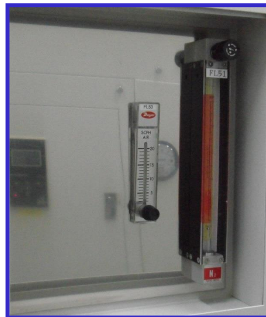
Flow Meter Panel (Exchange)
