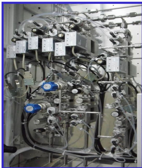
Gas Panel (Exchange)
